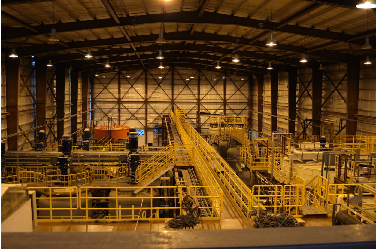
View of main lithium carbonate plant with primary and purification circuits.
