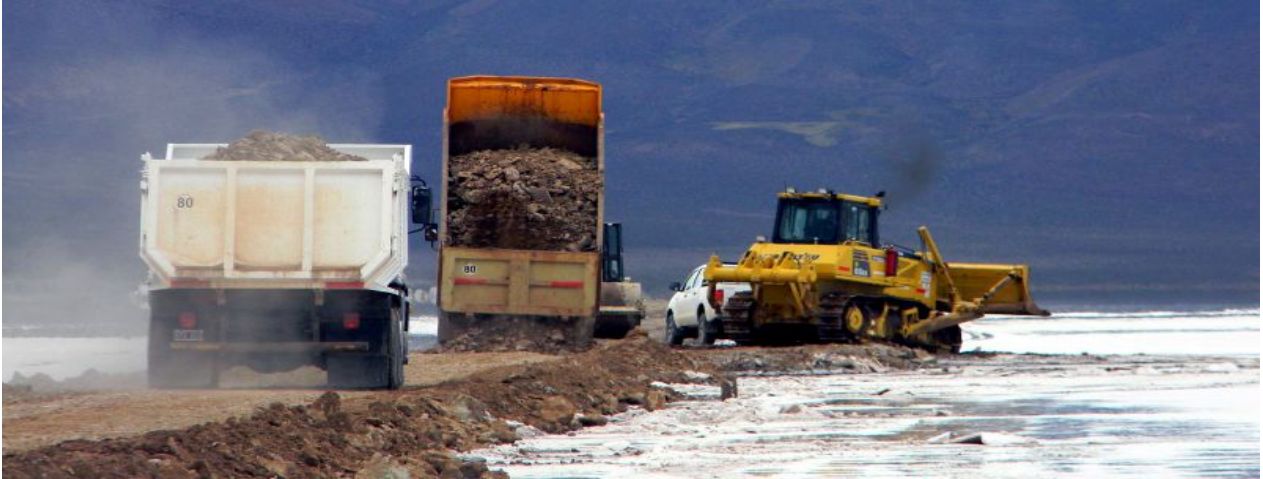
Figure 6: Construction of the road from the east side of the salar to the drilling area
